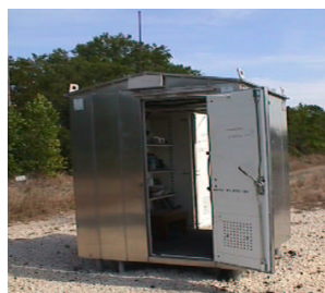
Data loggers in railroad wayside locations collect lightning and induction environments.
