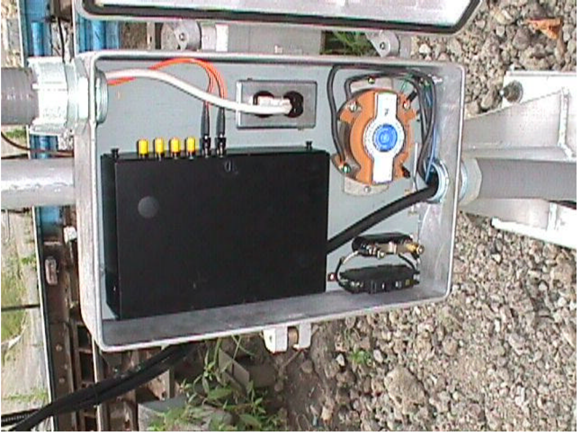
An Example of Improved AC Power Protection
