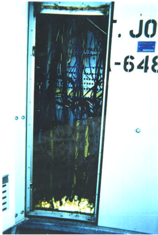
Back Door of a Bungalow Showing Black Dirty Wires and Blue Clean Wires Intermingled
